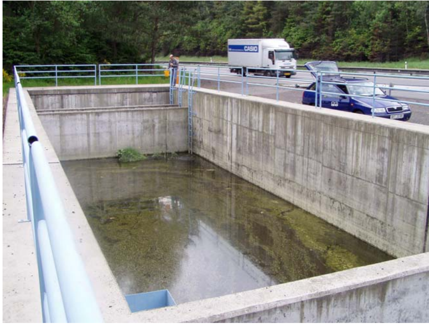
Figure 1: Profile on the storm water sediment basins (SWSB) on 61.5 km of D1
